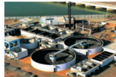
Sewerage Treatment Plant 10 MLD Commissioned, expandable upto 30 MLD
