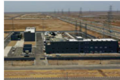
Power Substations 2 Substations (33/66 kv and 220 kv GIS) by Torrent Power
